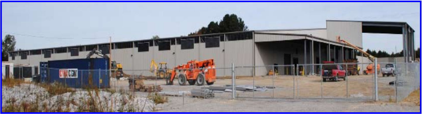
TRAXYS BUILDING. Shown above is the 105,000 SF industrial building under construction by Yellow Creek Port Authority. The building will be leased to Traxys. The company plans to begin installing equipment in January 2019.
